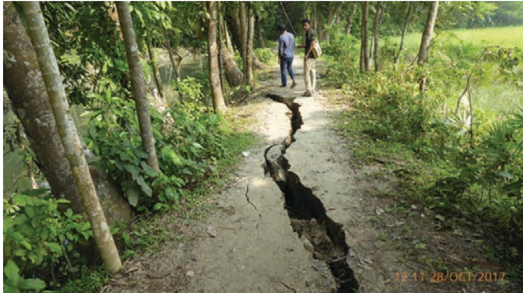
Water seepage from river (left) caused road collapse
